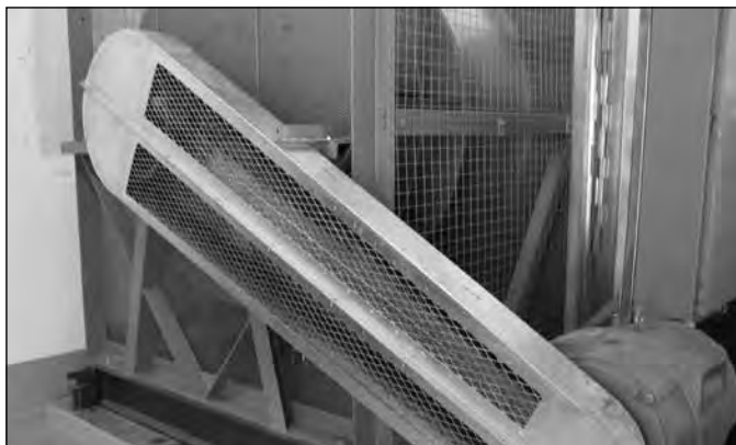
A properly guarded belt drive
